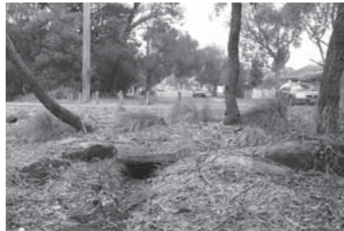
An extensive system of stormwater drains exist throughout Maroondah requiring monitoring, maintenance and renewal. Council's program for this year will see upgrade works for Georges Road stormwater and the second stage of Bridget Court works as part of the total drainage budget of $760,000.
