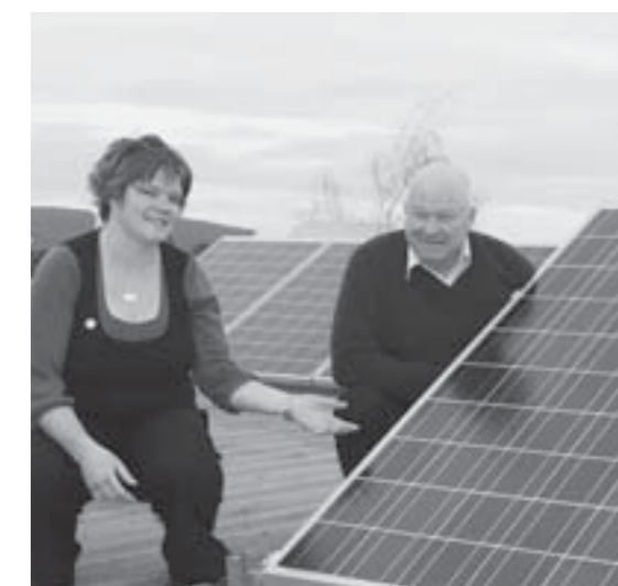
Mayor of Maroondah, Cr Peter Gurr and Rebecca Paslow, one of Council's Environment Planners, inspect the solar energy panels installed on the roof of the Braeside Avenue Civic Offices. The solar energy system offsets the energy consumed by a water pump, which is connected to a newly installed 173,000 litre rainwater tank to be used for toilet flushing throughout the building.
